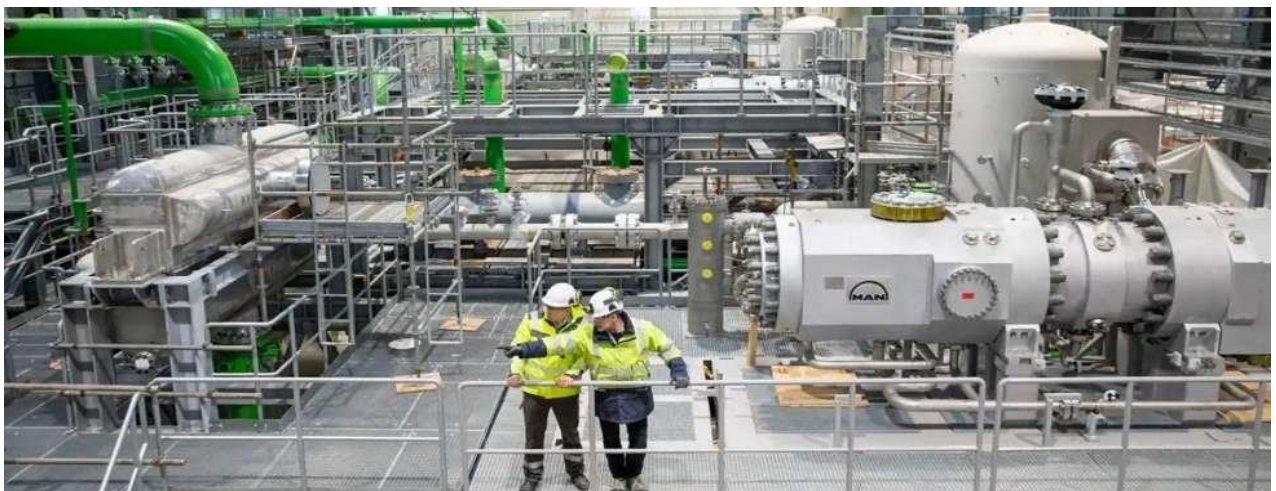
Balance of Plant in the industry for large capacities up to 1000 MW.
